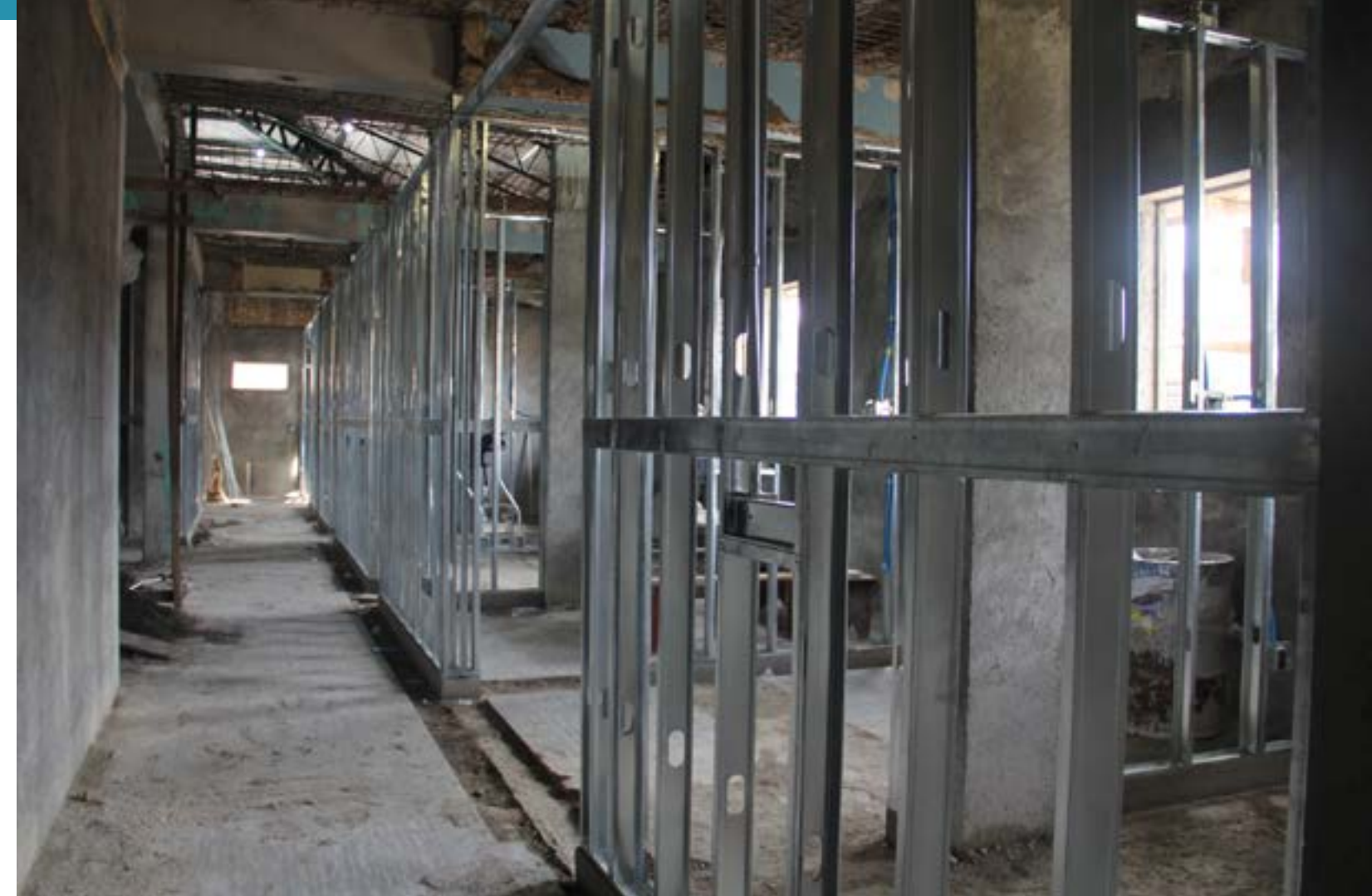
Construction of the Public Health Center is underway, showing a brand new roof and the beginnings of new walls.
