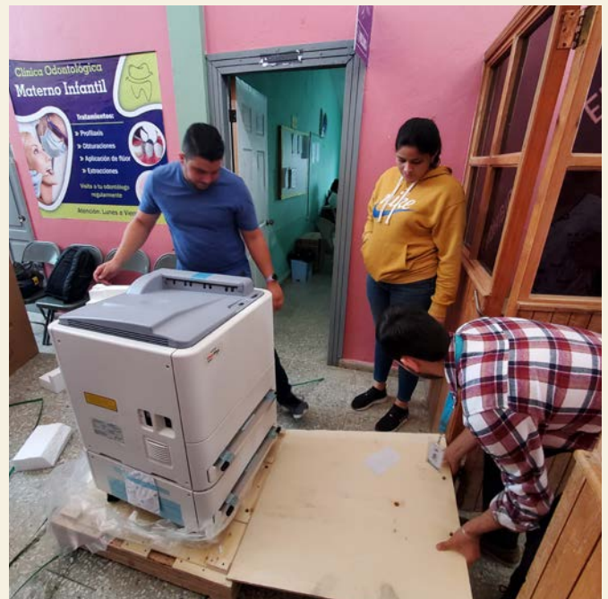
Installation of x-ray equipment at the maternal health clinic in Corquín, Copán.
