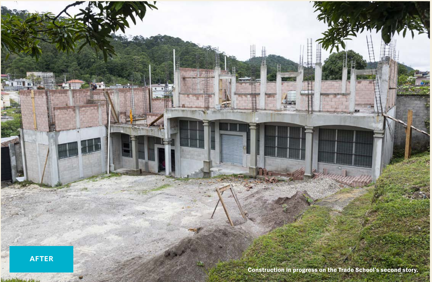
Trade School prior to the construction of the carpentry and welding areas.
